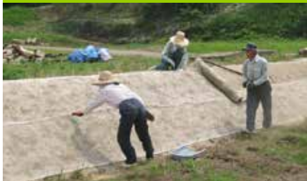
The Zoysiagrass Net-planting Technique (ZNET) facilitates the development of lawn levee banks.
