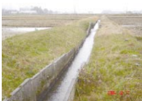
Fig.16 排水路の破損 Damage of drainage canal
