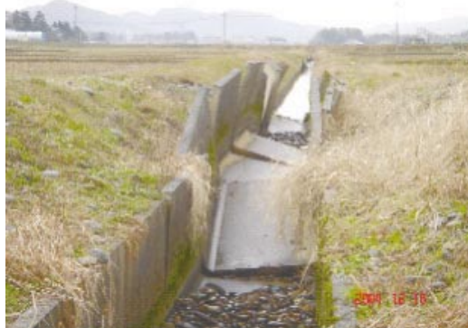
Fig.15 排水路の破損 Damage of drainage canal
