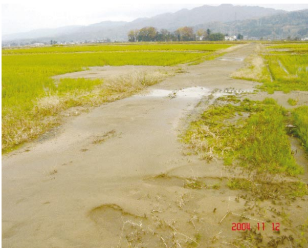
Fig.10 農道における噴砂 Sand blow in Farm road
