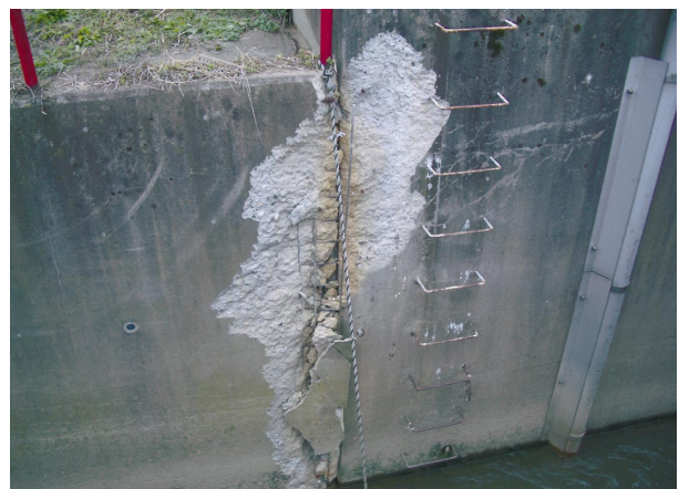
Fig.14 千谷放流工水路の継ぎ目部損傷（04.10） The joint failure in the wasteway canal
