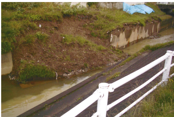
Fig.11 米沢川合流工付近の用水路側壁崩壊（04.10） Collapsing in canal left bank near a injection work of Yonezawa river
