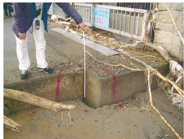
Fig.7 取水ゲート門柱基礎と護岸床との段差 (04.10) A difference level between a pier base and revetment base
