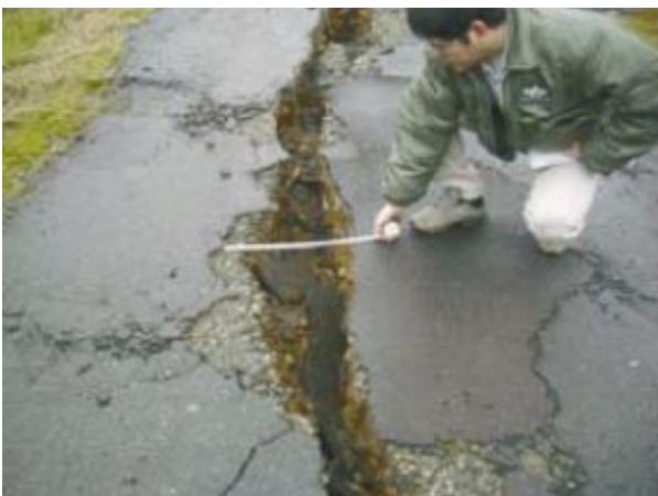
Fig.26 圃場内支線農道路面の亀裂(04.10) Cracking on the lateral farm road surface
