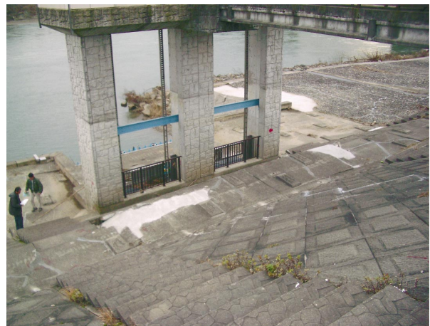
Fig.27 小千谷頭首工補修状況(04.12) A repairing situation in revetment of Ojiya Headwork
