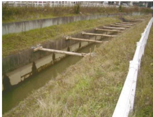
Fig.28 コンクリート水路の損傷と応急対策(04.12) Damages in the concrete retaining wall canal and emergency measures
