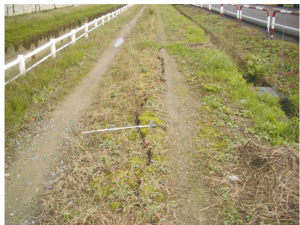
Fig.8 1号幹線水路右岸天端上の亀裂(管理用道路上)(04.10) A cracking on the maintenance road surface of right bank in No.1 main canal
