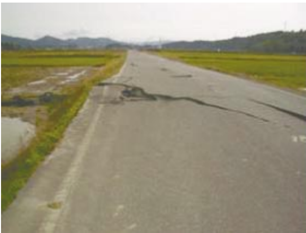
Fig.25 圃場内の農道(幹線)の道路面の損傷(04.10) Cracking on the trunk farm road surface
