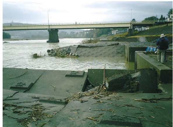
Fig.6 取水上流取入れ口護岸の損傷 (04.10) Damages of the intake revetment in Ojiya Headwork
