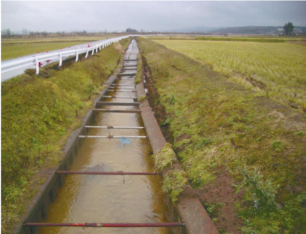
Fig.24-2 幹線排水路(鋼矢板)側部の変形(その2, 04.12) Inclining of the side wall in main drainage canal (steel sheet-pile)
