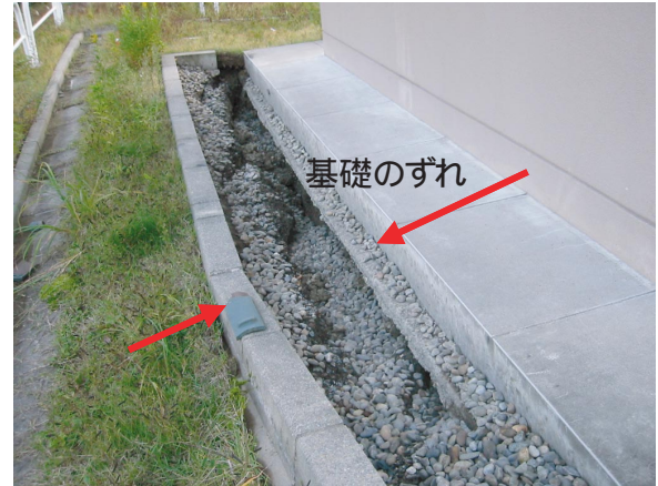
Photo 14 管理棟基礎のずれ Slide of footing of the inspection building at Tsuboyama dam
