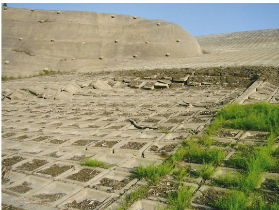
Photo 3 上流斜面の変状 (部分) Damages on the upstream slope (in detail) at Kawanishi dam
