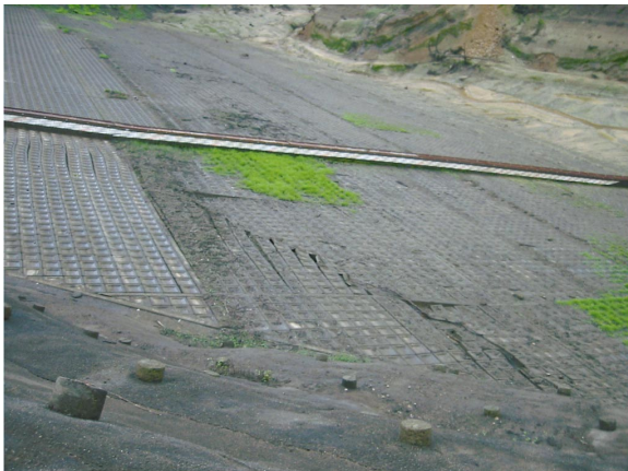
Photo 2 上流斜面の変状 (全景) Damages on the upstream slope (overall view) at Kawanishi dam
