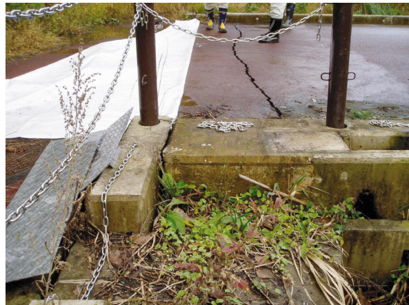
Photo 15 洪水吐取り付け部での段差 Different settlements and cracks at connecting part between the embankment and the spillway at Chofukuji dam
